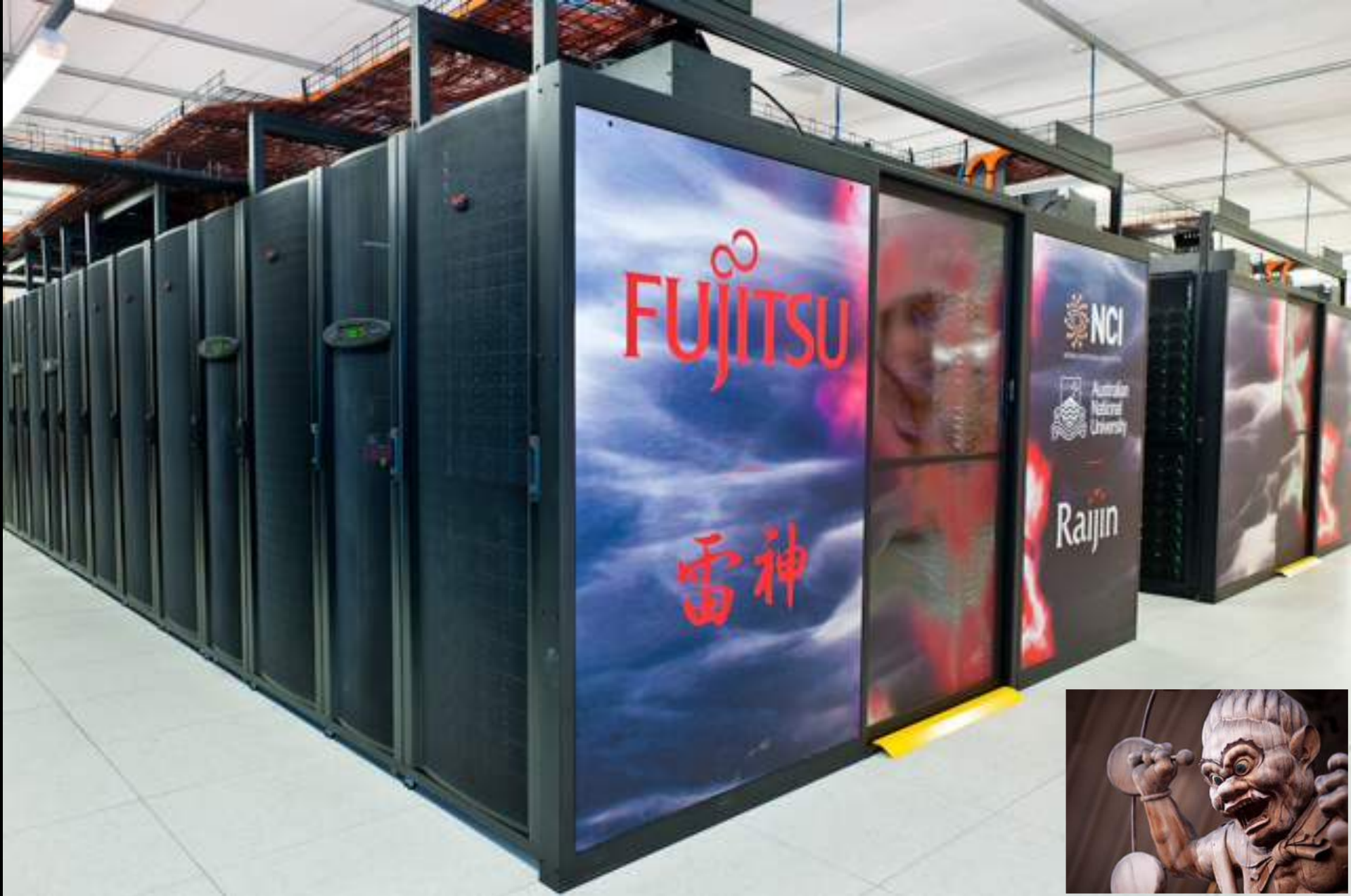
“Raijin” (named after the Shinto God of thunder, lightning and storms) National Computational Infrastructure, ANU, Canberra, Australia
