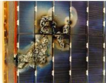
Dangerous Particles to Electronics and People
