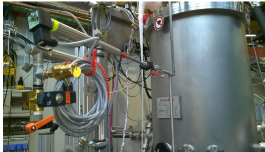
Automatic He-transfer for 7T horizontal cryomagnet: High Field Diffractometer UE46_PGM-1, HZB
