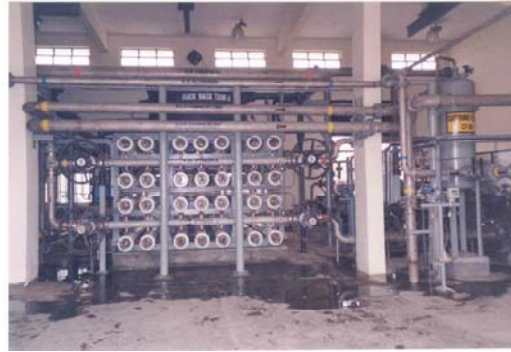
Fig.6 View of SWRO membrane modules at Kalpakkam
