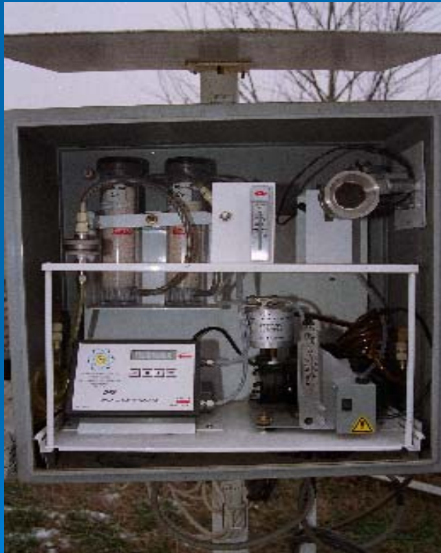
Fixed air monitoring station
