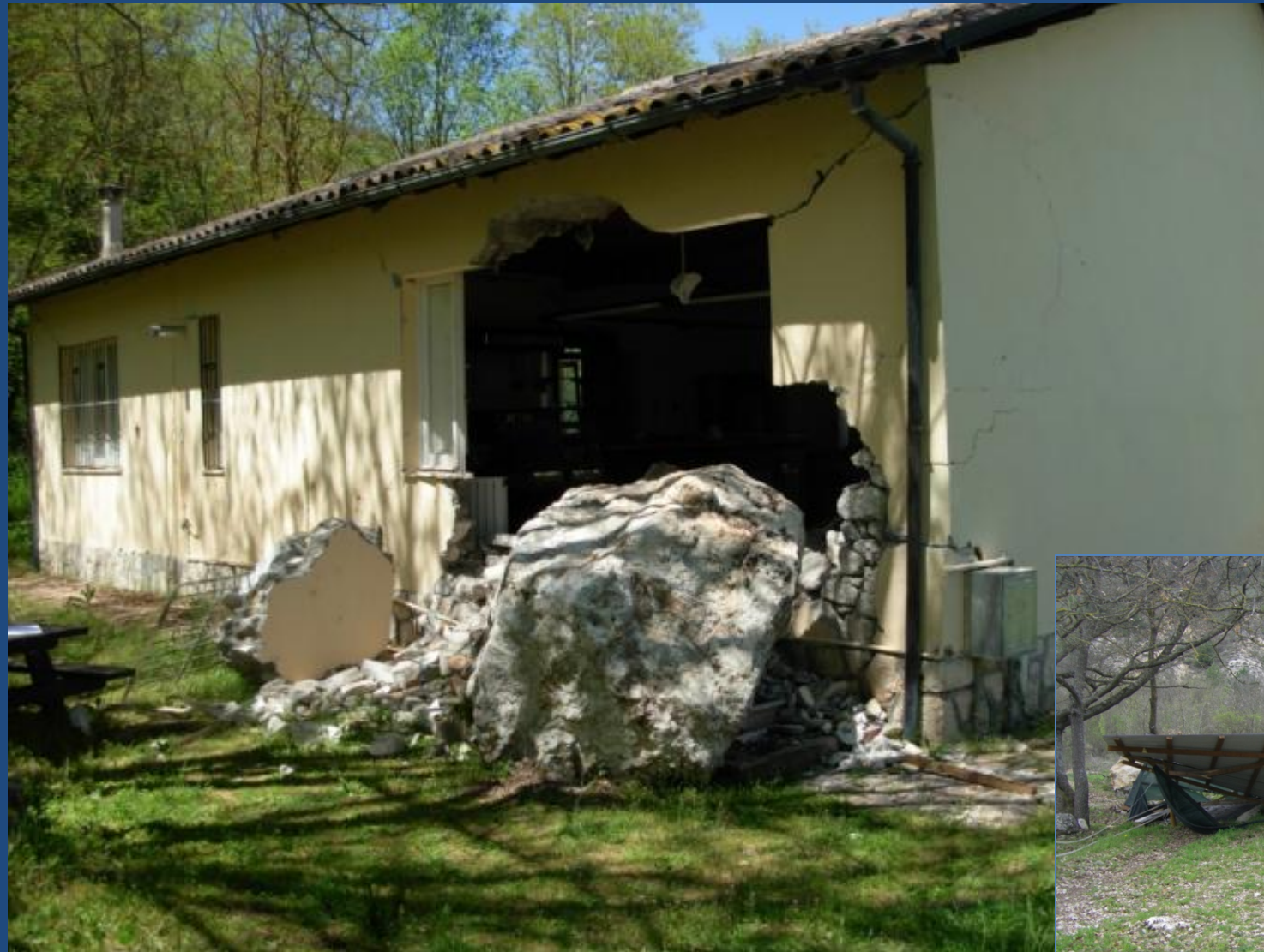
Rock fall at Stiffe
