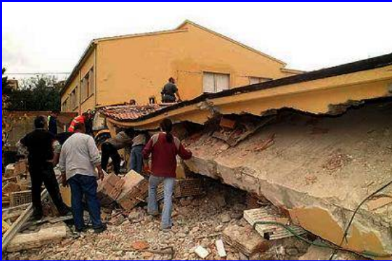
October 31, 2002: 27 children die due to the collapse of the F. Jovine primary school at San Giuliano di Puglia (Italy)
