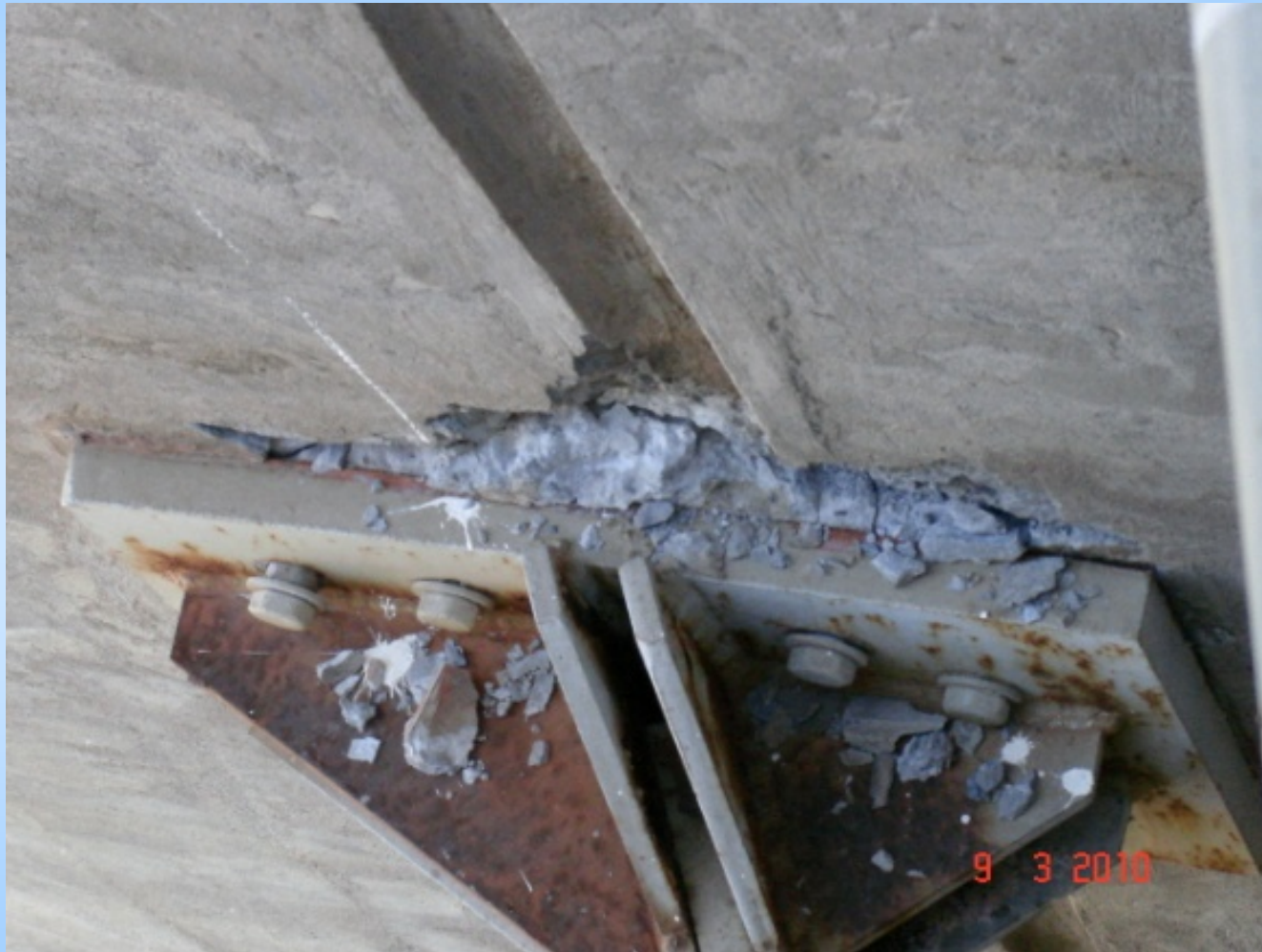
LOOSE CONCRETE IN ANCHOR BOLTS
