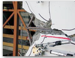
Identification of insufficient seismic detailing, tall pier A40, buckling of longitudinal reinforcement at h = 3.5m
