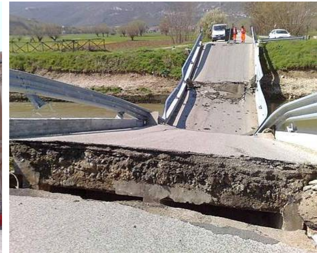
Failure of a bridge
