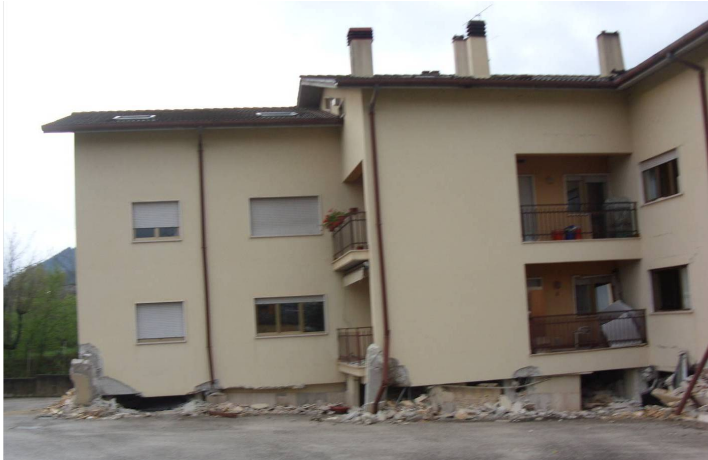
Building in via Dante Alighieri 2 After earthquake
