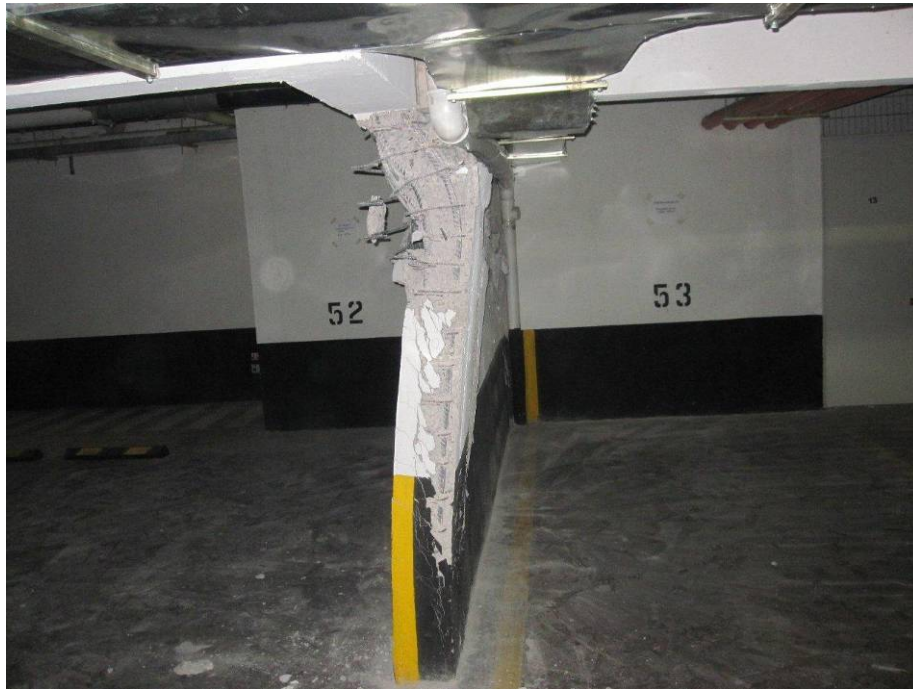
Santiago, Edificio Emerald. Severe damage in the basement's shear walls.
