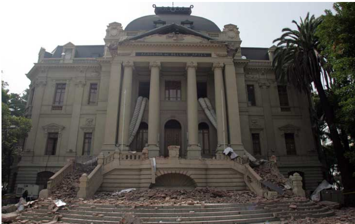
Damage to monument
