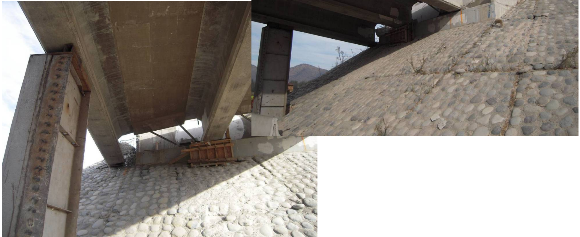
Ruta 5, Paso Inferior de la Merced. Loss of support
