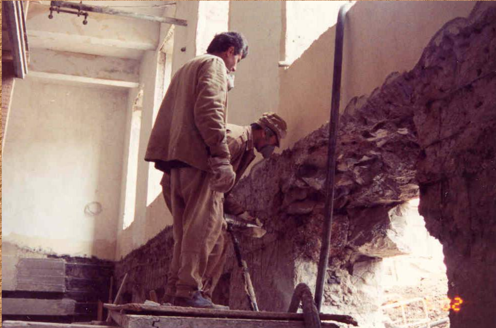
The case when the opening has the part of the existing wall above it
