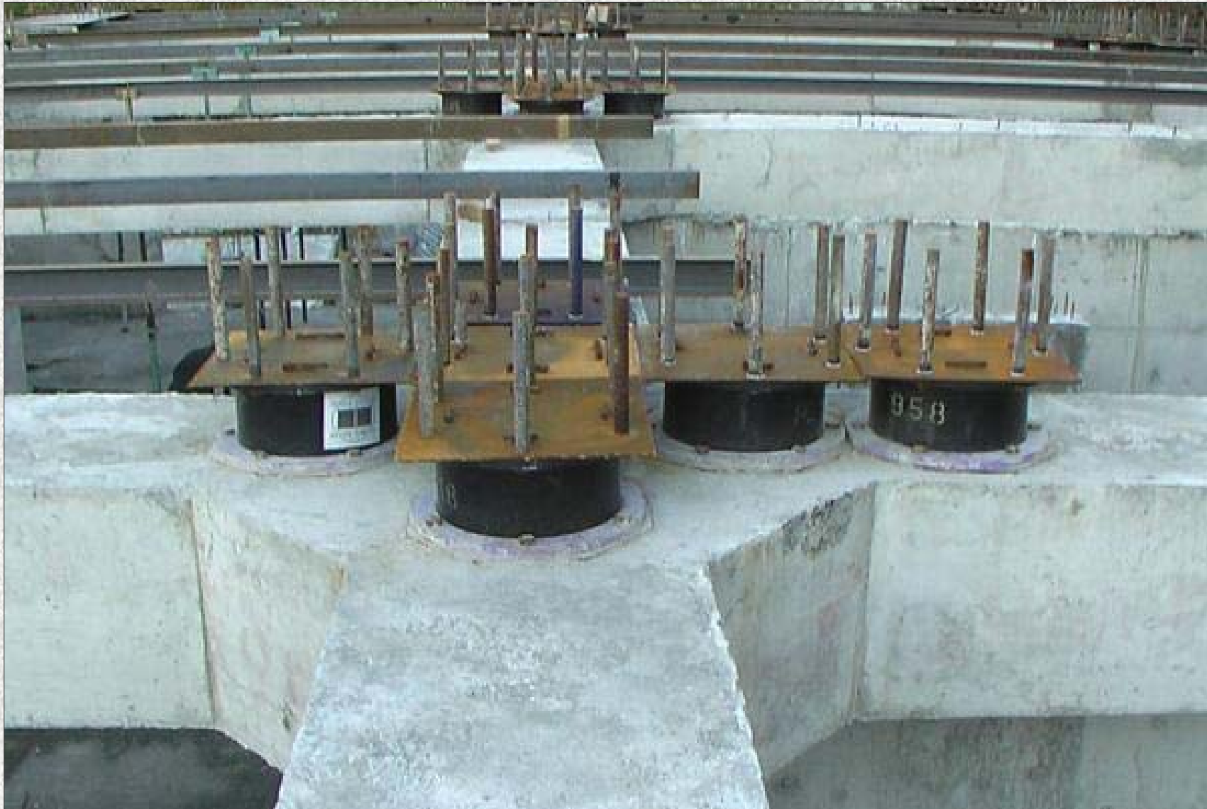
Examples of installation of different quantities of rubber bearings under the columns of base isolated buildings
