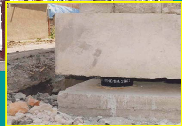
Retrofitted by base isolation existing 3-story building of school #4 in Vanadzor. Project financed by “CARITAS Switzerland” in 2002
