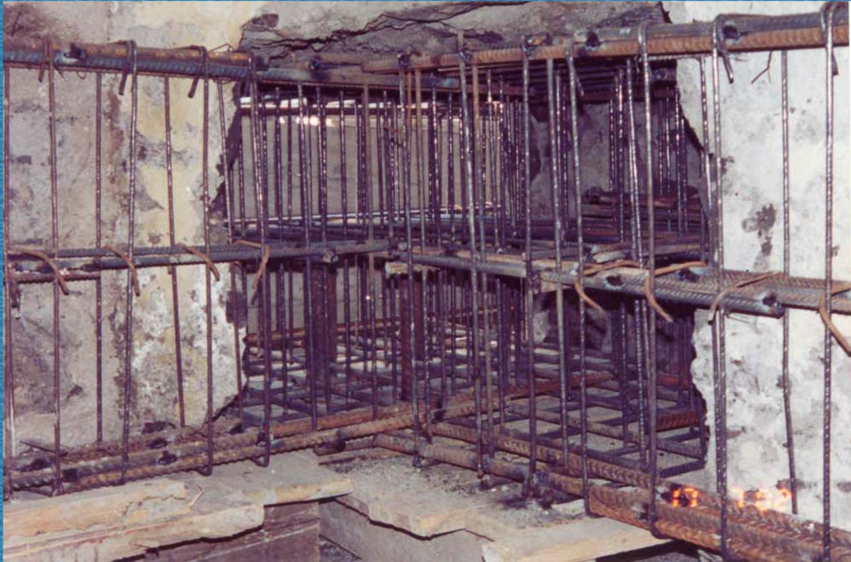
The view of the upper reinforcement frame installed in the opening together with the isolator upper socket after casting the concrete of the lower pedestal
