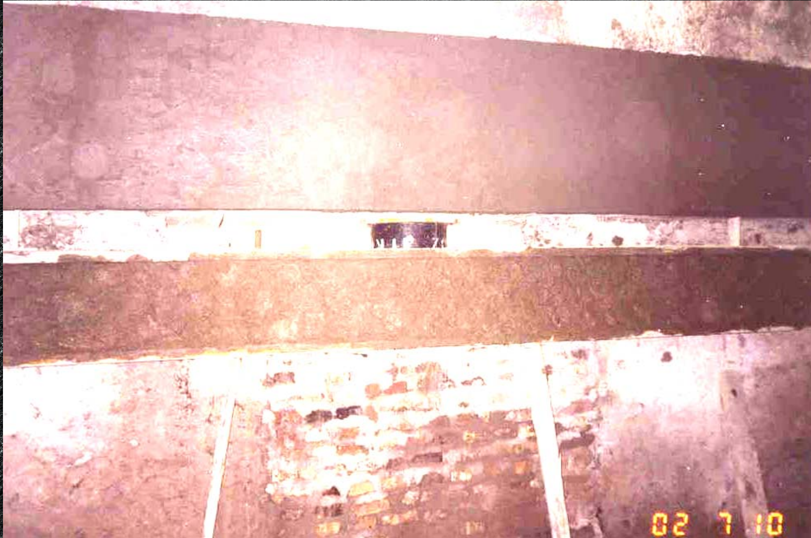
The view of a two-stage system of R/C continuous beams, which separate the building from its foundation and create the seismic isolation system
