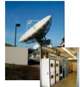
6 Ground Earth Stations
