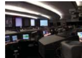
2 Operational Control Centers
