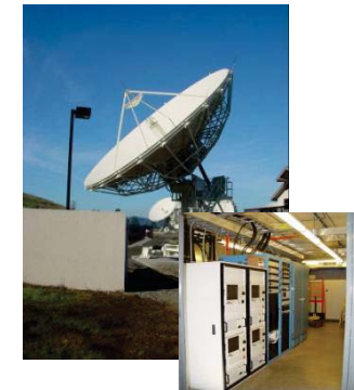
6 Ground Earth Stations
