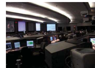
2 Operational Control Centers
