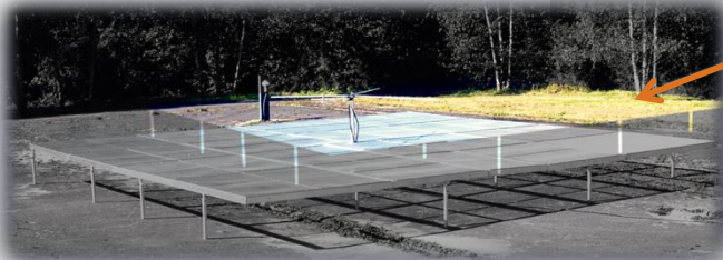
Dedicated transmitter in Dourbes
