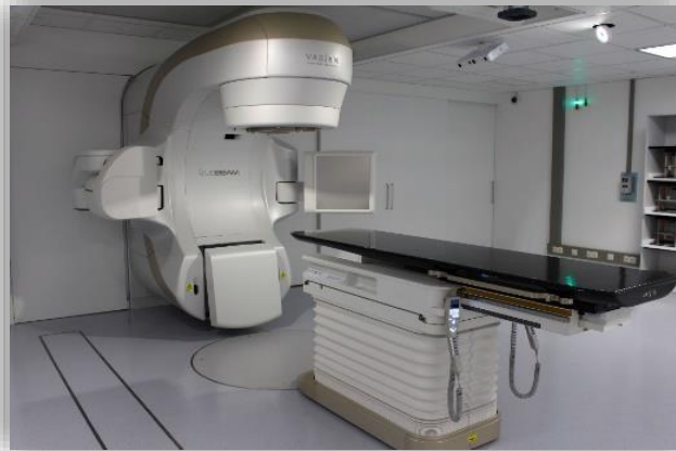
Linear Accelerator Facility
