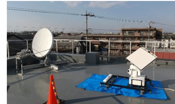
Gateway station and VSAT station
