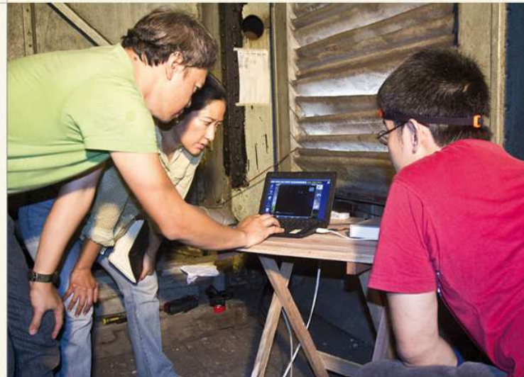
Dry run: the technical team is glued to the monitor as the camera is lowered to the column base, which has never been seen since construction in 1891. From left: Engineer Reggie Mercado, executive director Tina Paterno, and architect Jonathan Dangue
