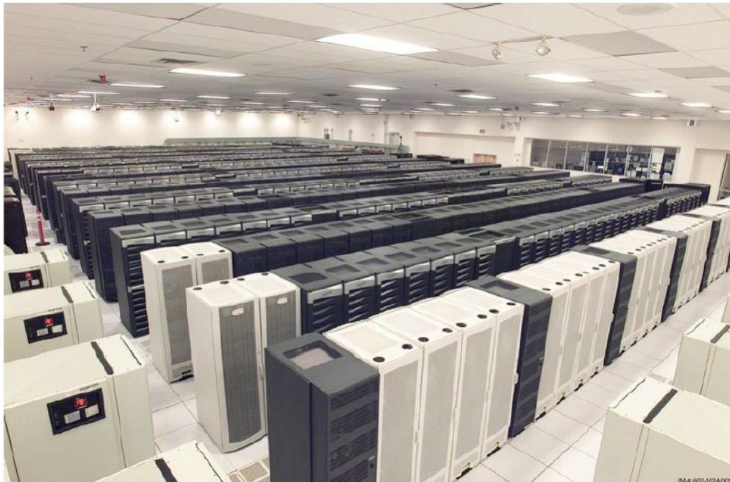
Figure 5. This shows a large high-performance computer at Los Alamos National Laboratory. This is typical of large data centers, which can be vulnerable to thermal neutrons causing SEE.
