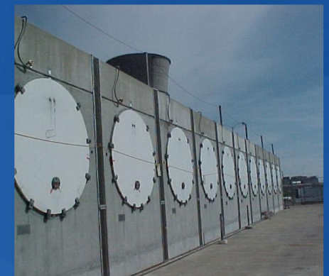
Horizontal Storage Module
