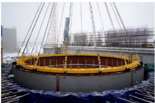
The lower tier of the enclosing structure was immersed in the reactor shaft (December 2023)
