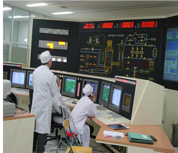
Main control room
