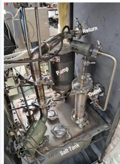
Inside Enclosure Furnace
