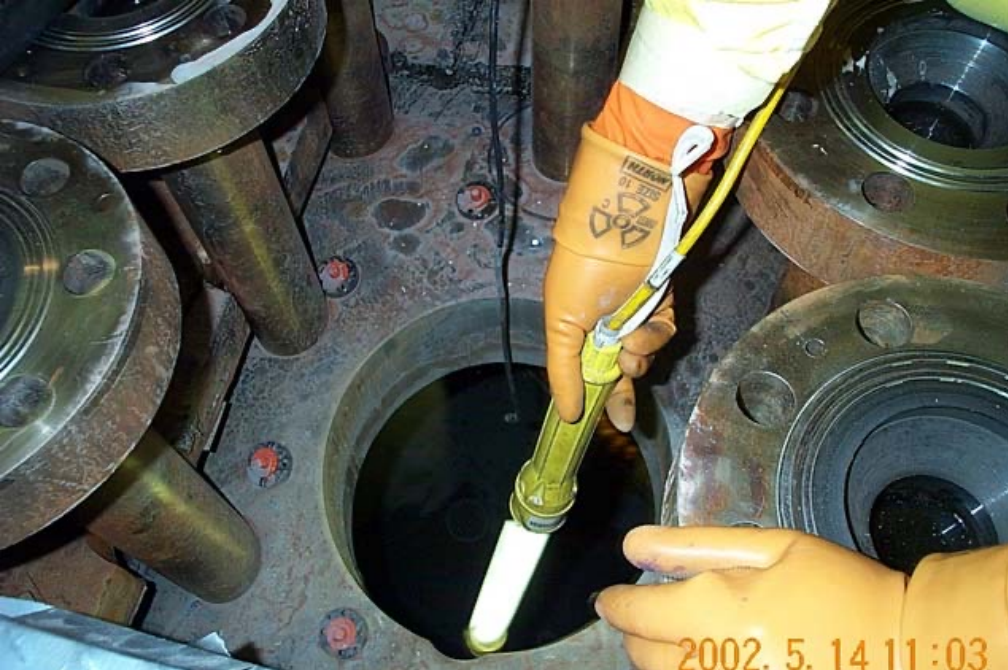
Top View - Nozzle #3 Removed
