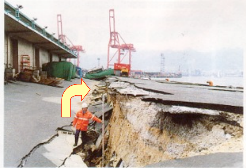
Photo 11. Damaged caisson type quay walls at Port Island in Kobe Port
