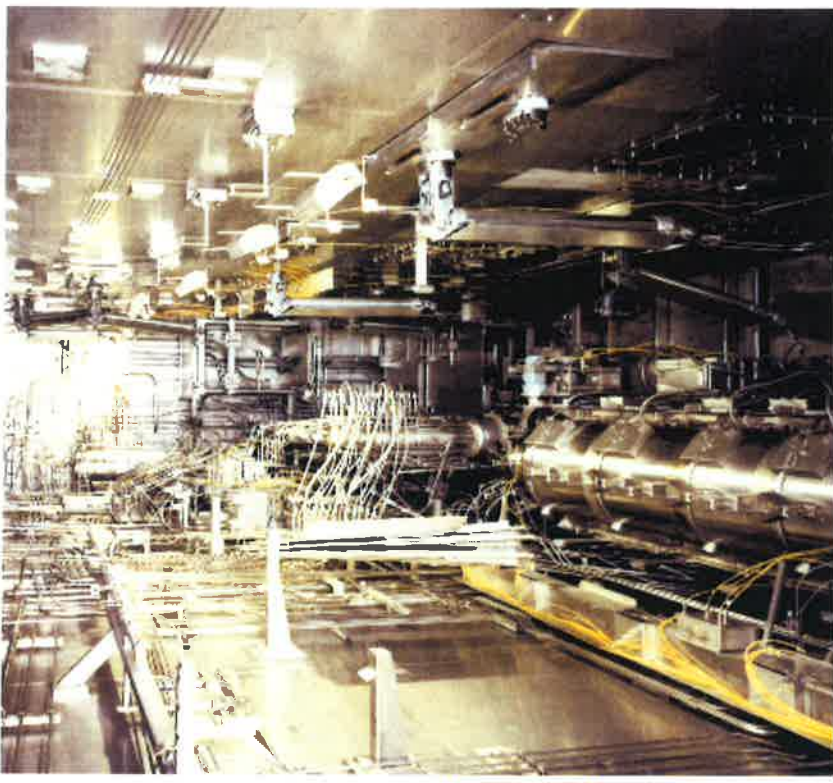
5 vitrification lines in operation at AREVA La Hague Facility
