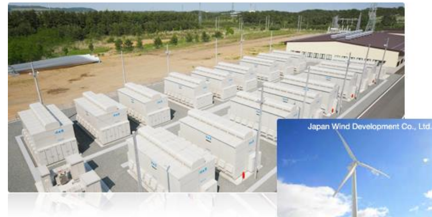
Exemple: 34 MW NAS alongside 51 MW Wind Farm Courtesy of NGK Insulators – Japan)
