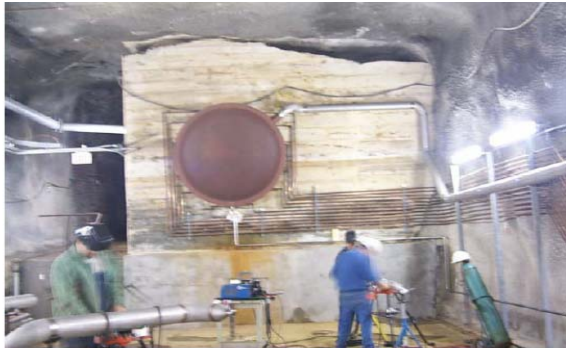
Decay Pipe Endcap at Absorber Hall
