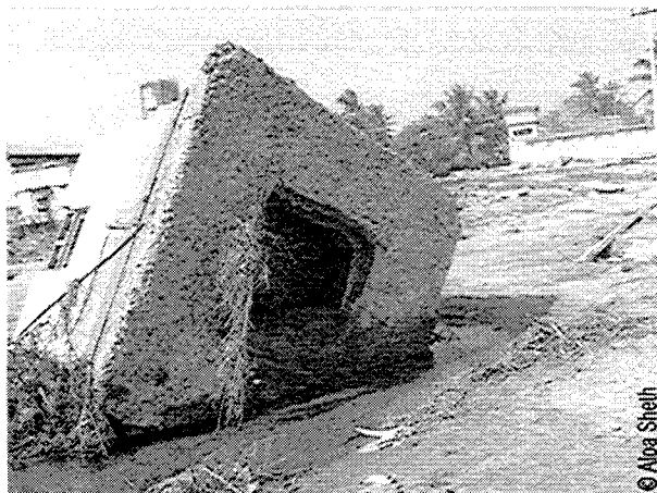
Overturning due to scouring around the foundation, pump house
