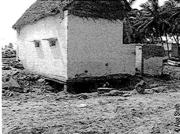
Scouring below the foundation of the house
