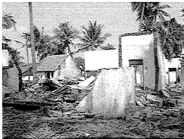
Collapse of load bearing walls
