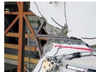
Identification of insufficient seismic detailing. tall pier A40, buckling of longitudinal reinforcement at h = 3.5\text{m}
