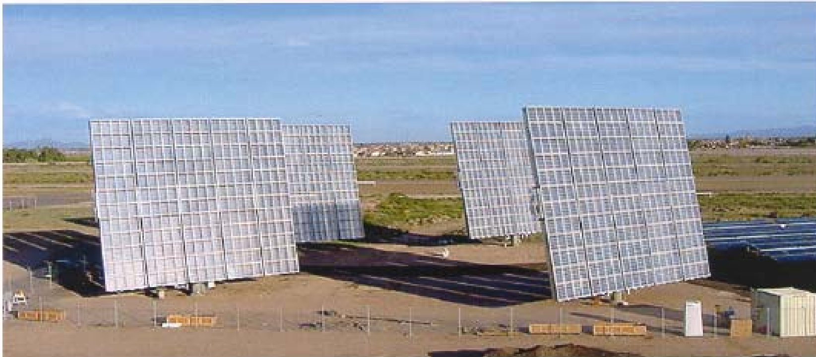
Figure 1: Amonix/APS 100 Kilowatt High-Concentration PV Installation in Arizona, USA
