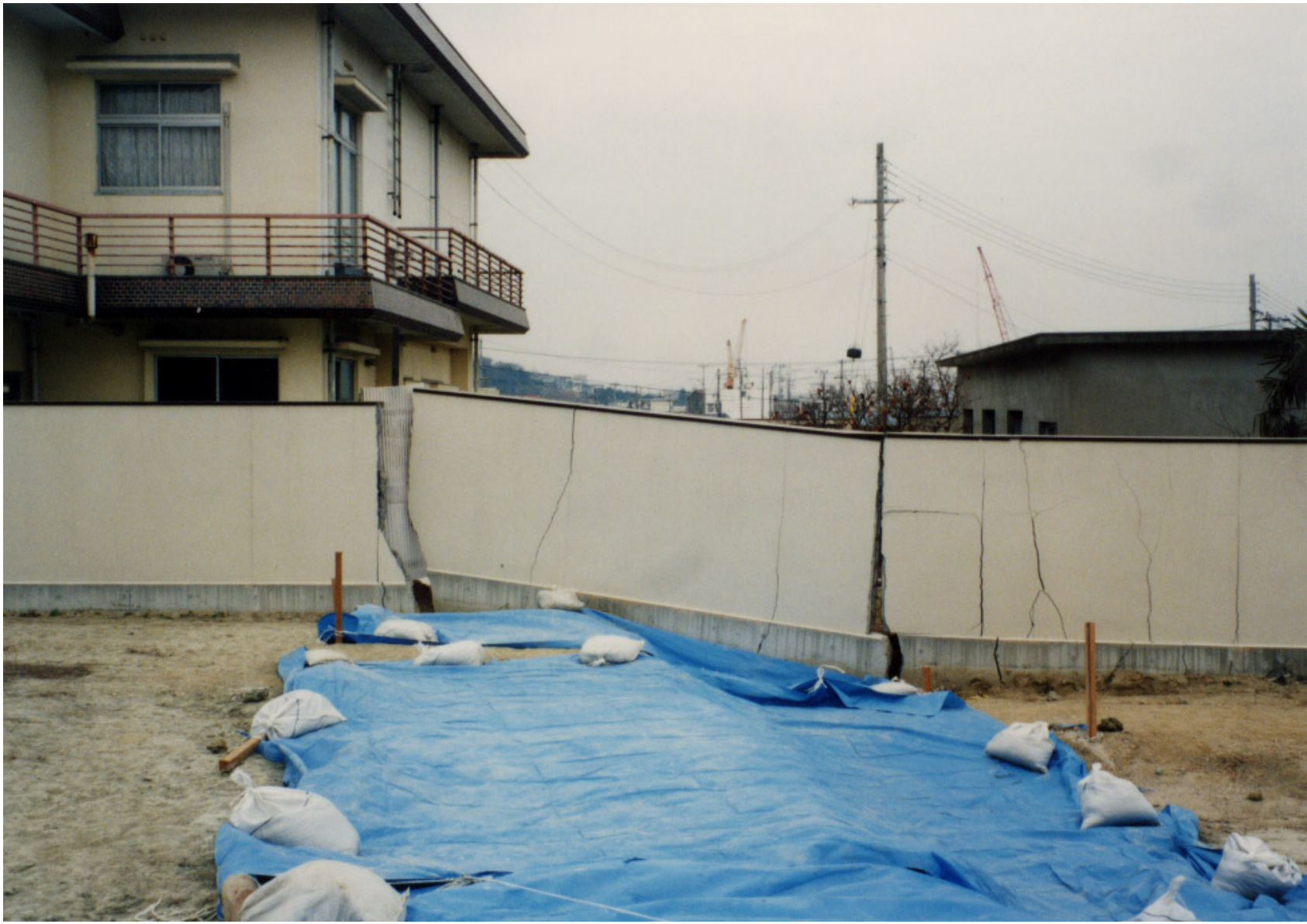
Broken wall by the fault displacement
