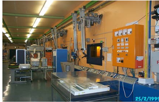
Hot Cell Laboratory for the characterisation of spent nuclear fuel
