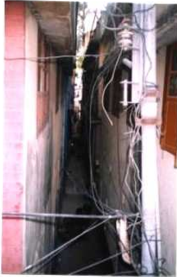
Risky Electrical Wiring
