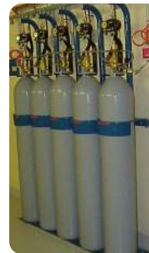
CO 2 fire extinguisher
