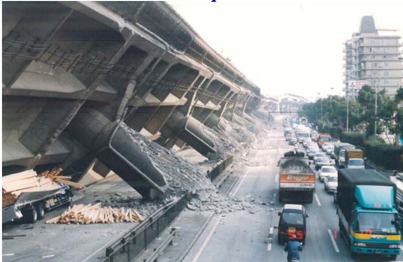
Collapse of Hanshin Expressway Running near Source Area
