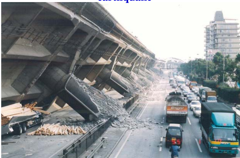
Collapse of Hanshin Expressway Running near Source Area
