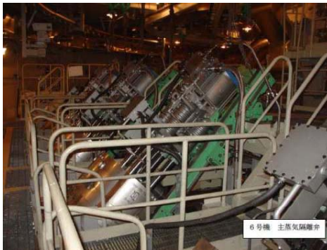
Inside view of unit 6's equipment (around main steam isolation valves)
