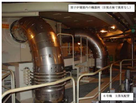
Inside view of unit 6's equipment (around steam piping)
