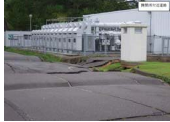
Road damage near switch yard
