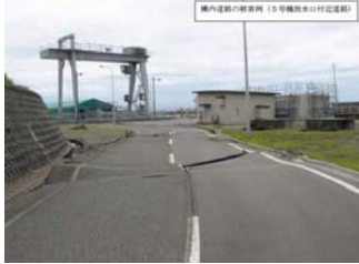
Road damage near water discharge
