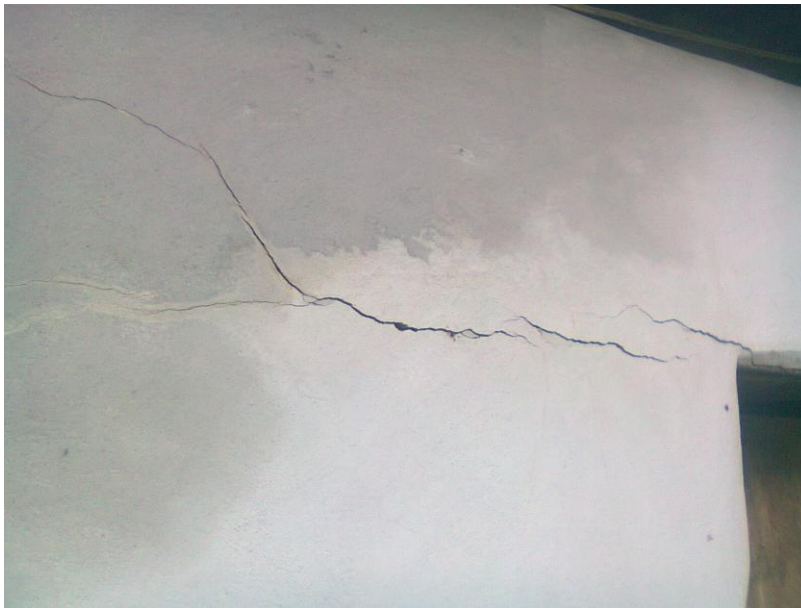
Figure 7. Type of the damage observed in adobe constructed houses in Salvadoran border houses.
