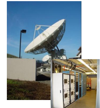
6 Ground Earth Stations
