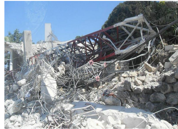
Damaged communication infrastructures
